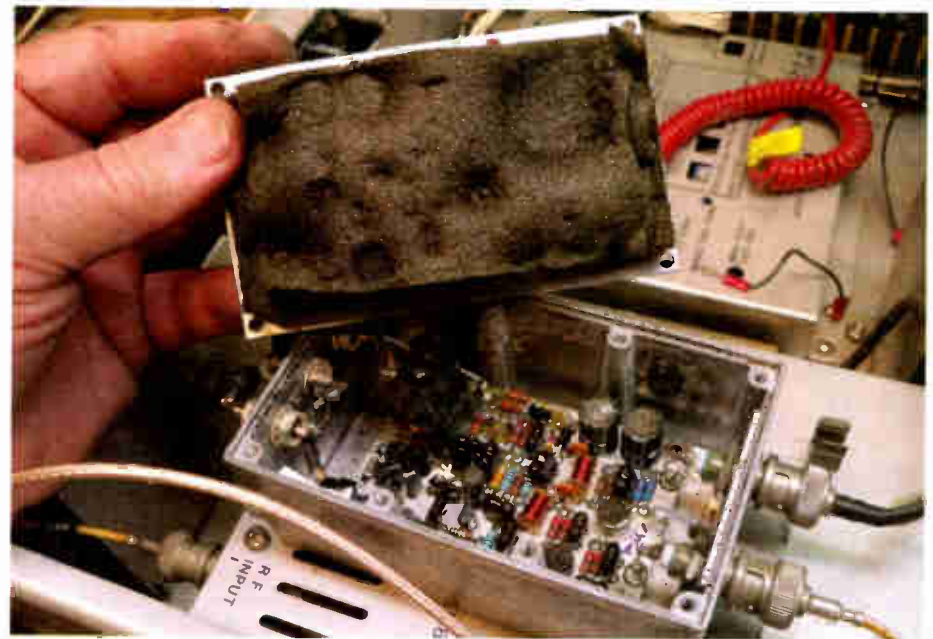
Fig. 2: Inside the exciter module where electrolytic capacitors were replaced.
