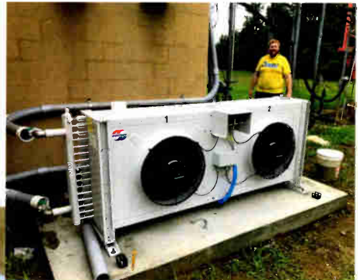
Fig. 3: Nathan Briton Smith, the CE at WYCT(FM), Pensacola, Fla., stands behind the heat exchanger outside the transmitter building.
