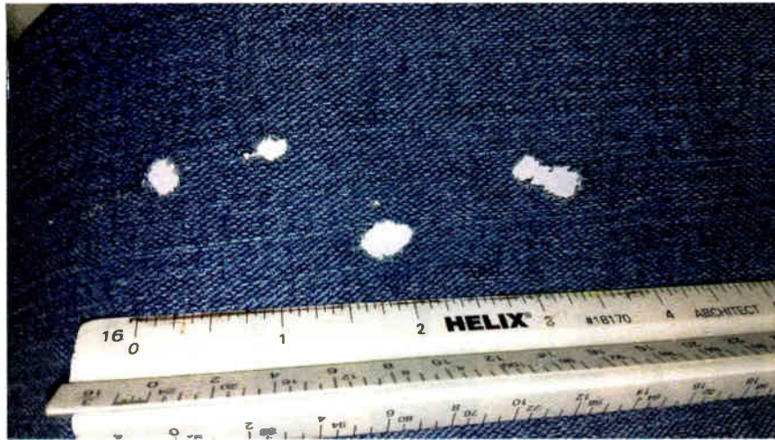
Fig. 1: Battery acid spill from "sealed" UPS batteries.
