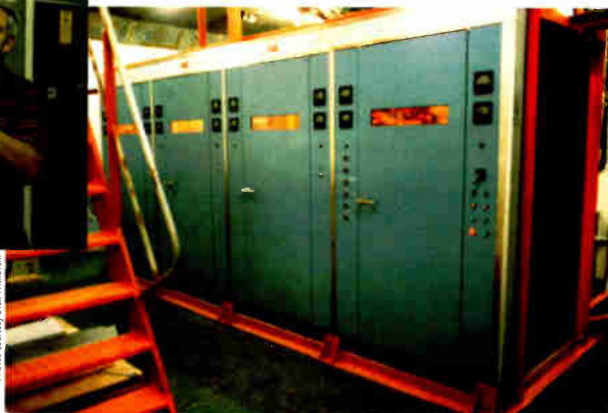
50 kW RCA Ampliphase transmitter on Caroline
