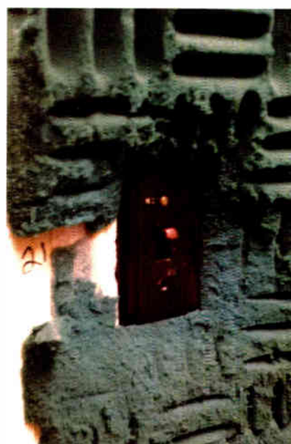
Fig. 3: How would you handle this problem of deteriorating foam sound-proofing?
