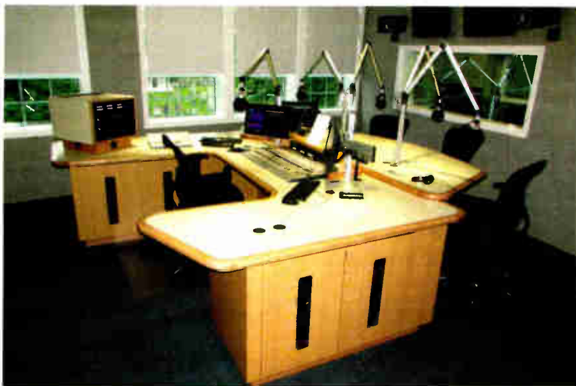
A Studio Technology project at Binnie Media. Note the single equipment rack set off to the side and computer equipment far more centrally located.
