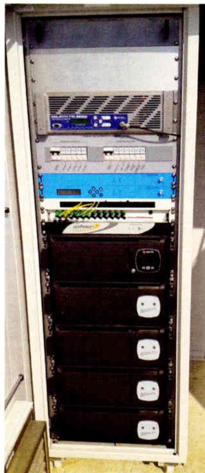
A typical STIC site setup. Note the Audemat Silver in the middle of the rack. WorldCast also provided the Ecreso Goliath transmitter amplifier at the top of the rack.
