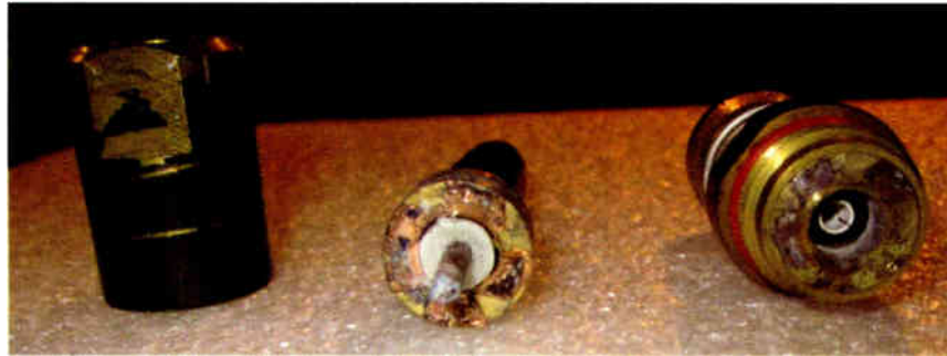
Fig. 1: A corroded RF connector, sealed only with electric tape.
