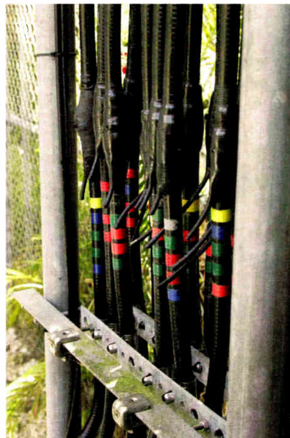
Fig. 5: Not much left of these cable ground kits, hacked off by copper thieves.
