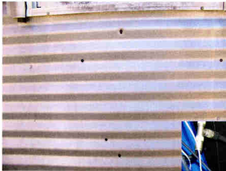
Fig. 1: Bullets penetrated this transmitter building.
