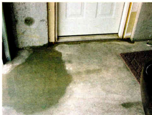
Fig. 2: Be alert to possible water damage as snow melts and spring rains arrive.
