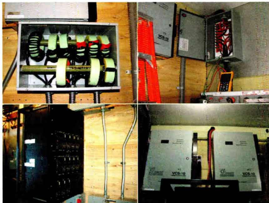
Top left: Static suppression coils on the turbine power cables. Top right: The Exeltech inverter. Bottom left: The DC source center is the heart of the DC bus in this 48 VDC system. Also visible are the top of the battery bank rack (lower right) and one of the three VCS charge controllers. Bottom right: The VCS-10 rectifies the voltage from the turbine and puts the power into the DC bus. One charge controller is needed per turbine.
