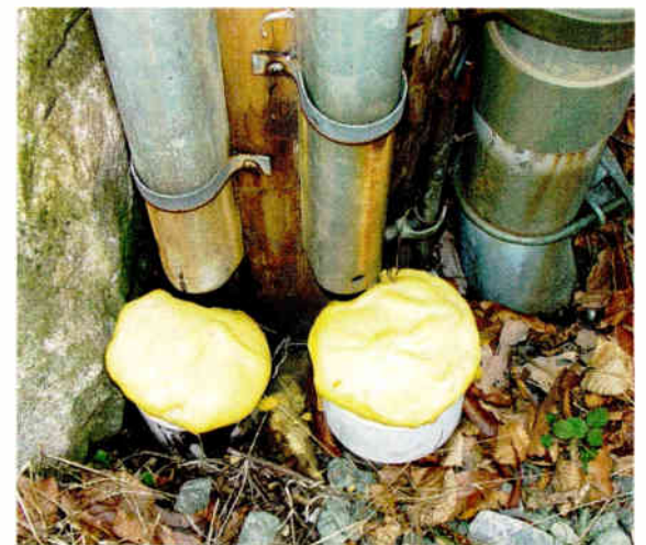
Fig. 4: Conduit at the transmitter site should be plugged. Expandable foam is used here.
