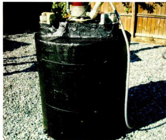
Fig. 1: Coat the base pier with tar to discourage copper theft.
