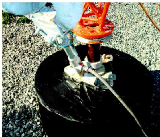
Fig. 3: A closeup of the top of the pier. The tar greatly reduces salvage value of the copper.
