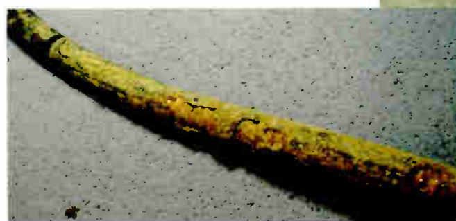
Fig. 2: A cable, buried in the sand, looks benign ...
