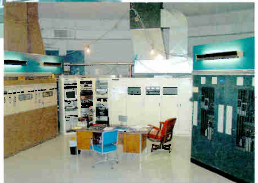
Fig. 2: A hood over the transmitter exhaust port is a better idea, as seen above the Harris transmitter, center.
