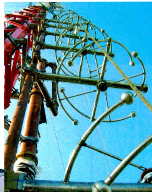
The two tetraplexed Dielectric systems are shown installed.
