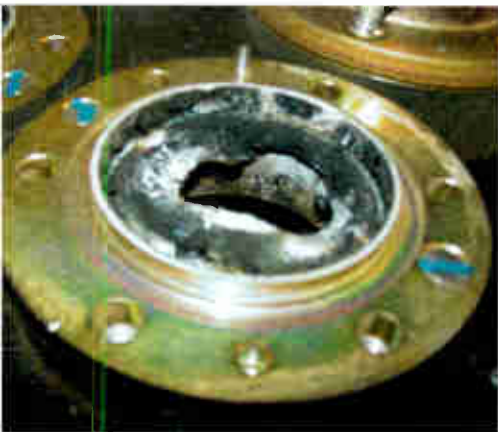
Fig. 3: Switching a transfer switch 'hot' causes this kind of damage.
