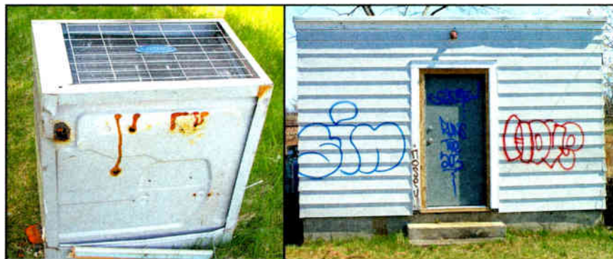
A damaged AC unit; graffiti on the generator shack.
