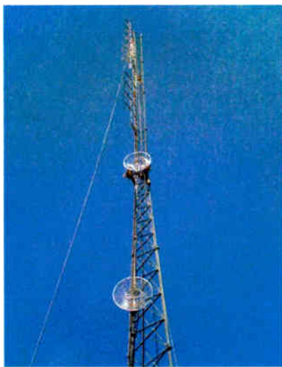
KHLX's new Jampro antenna is on top of this tower.
