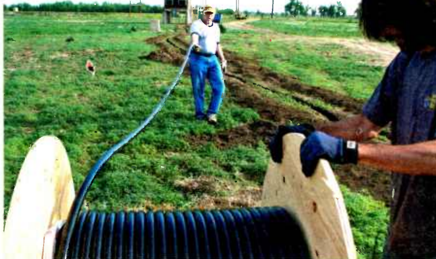
Assisted by Keith Peterson, the author pulls 7/8-inch transmission line off the spool.
