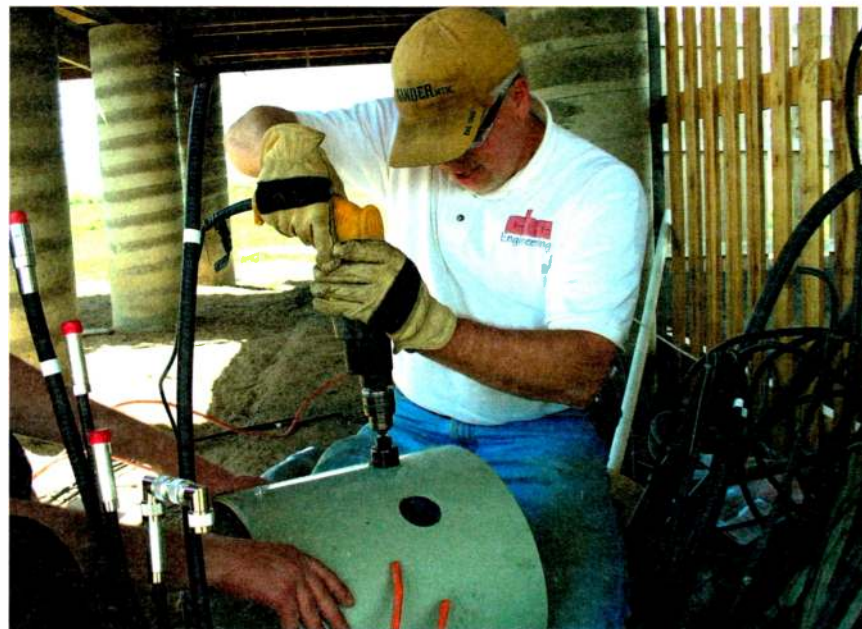
Drilling through the telco-style splice pedestal. Cable splices were made with connectors and 90-degree 'elbows.'
