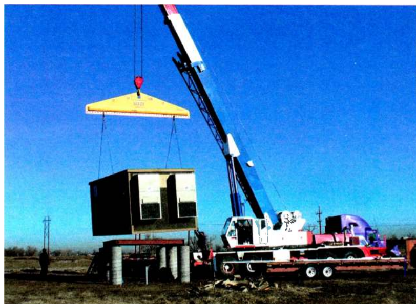
The 60,000 pound pre-fab concrete building is set in place on its elevated foundation with a crane.
