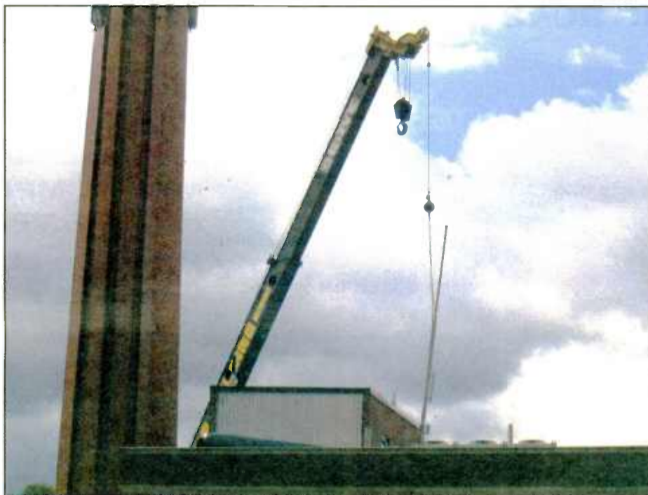
A cost not originally envisioned for this installation was the crane necessary to install a pole of the landlord's structural engineer's specifications. The presence of 'contingency funding' in the budget kept this from becoming a problem.
