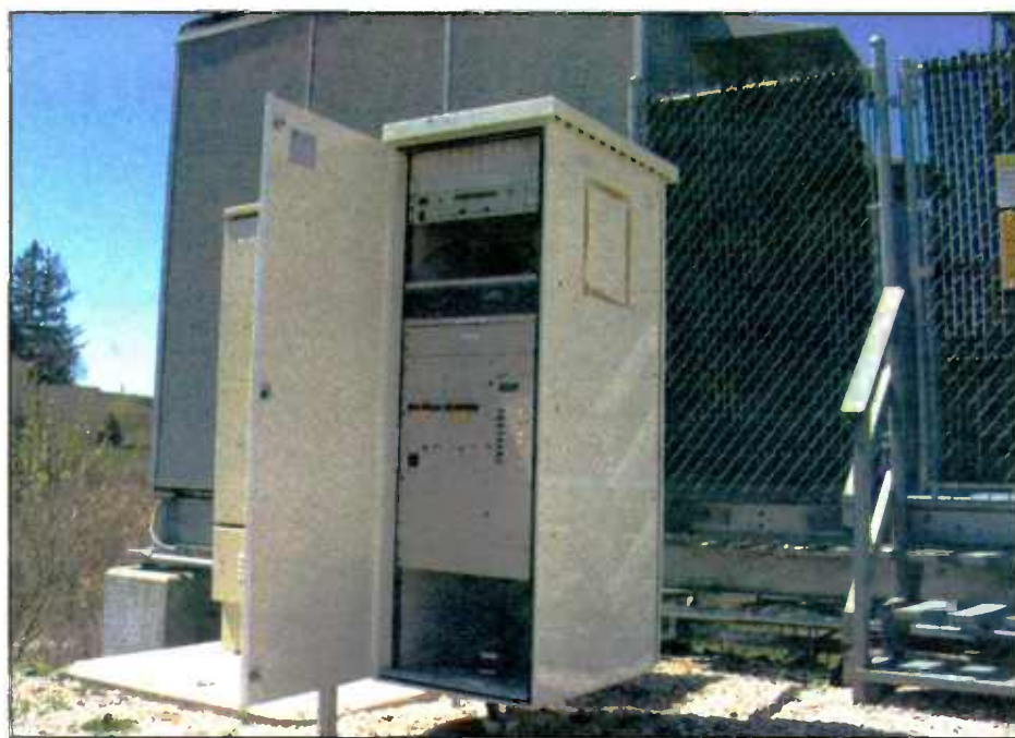
With its 600 watt TPO Broadcast Electronics transmitter, this cabinet required upgraded ventilation.
