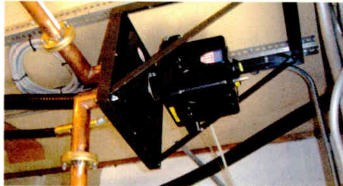
Fig. 1: Mounting switches? Bill Ryall's welded transfer switch brackets can speed the job.
