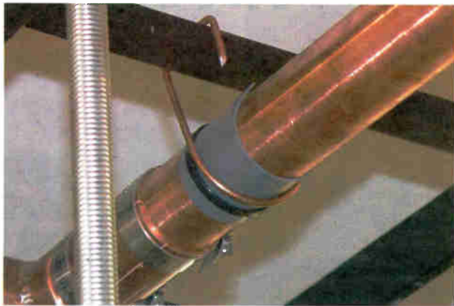
Fig. 3: Heavy-gauge copper wire can be used to temporarily hang lines, ensuring straight runs.
