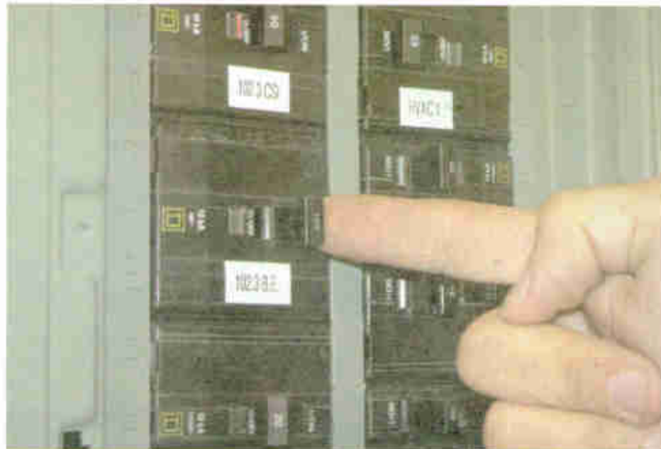
Fig. 1: A label placed directly on the breaker makes identification easier.
