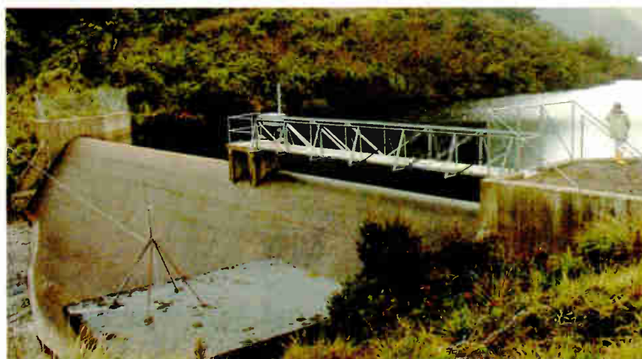
The Lake Loreto dam is one of three in HCJB's hydro system.
