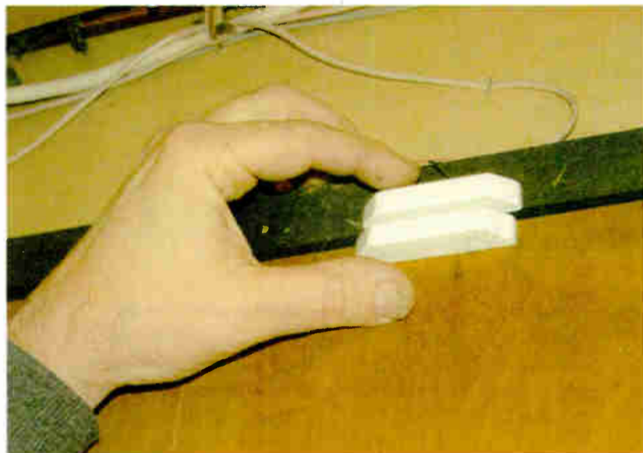
Fig. 2: A simple magnetic switch tied to the transmitter door alerts through the remote control.
