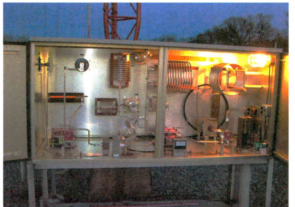
A look inside WPEN's ATU shows the 'station switch' contactor at left. There is a similar arrangement at each of the four towers. These contactors are controlled by a GPS clock system that connects the correct station to the tower at the licensed sunset and sunrise times each day.
