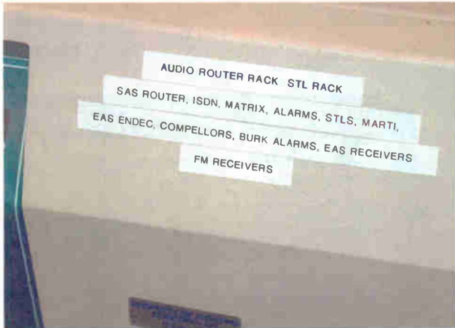
Fig. 4: For quick identification, label the circuits connected to your UPS.
