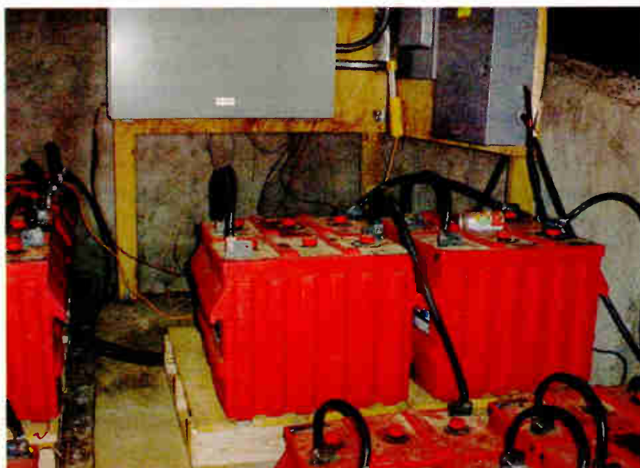
Part of the lead-acid battery bank charged by KTAO's solar array.
