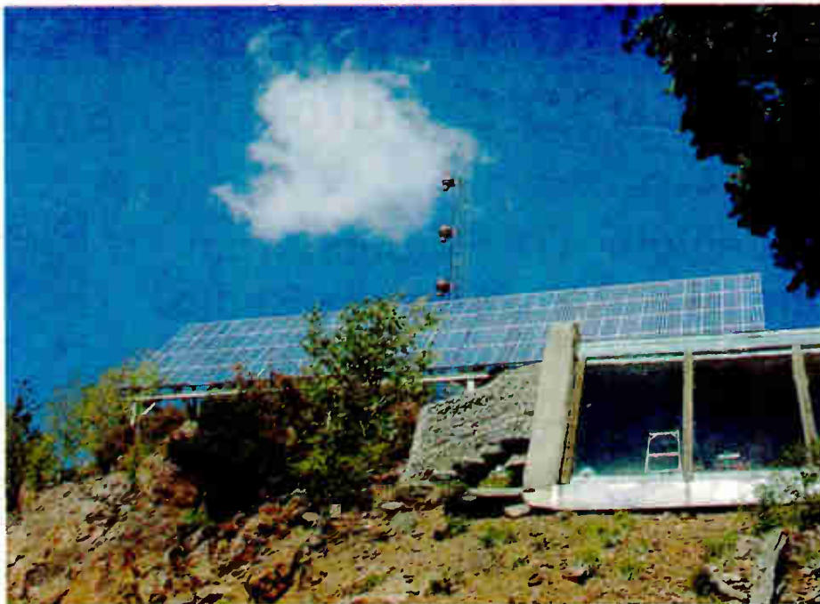
An array of 135 solar cells provided 100 percent of the power for KTAO's mountaintop transmitter site near Taos, N.M.
