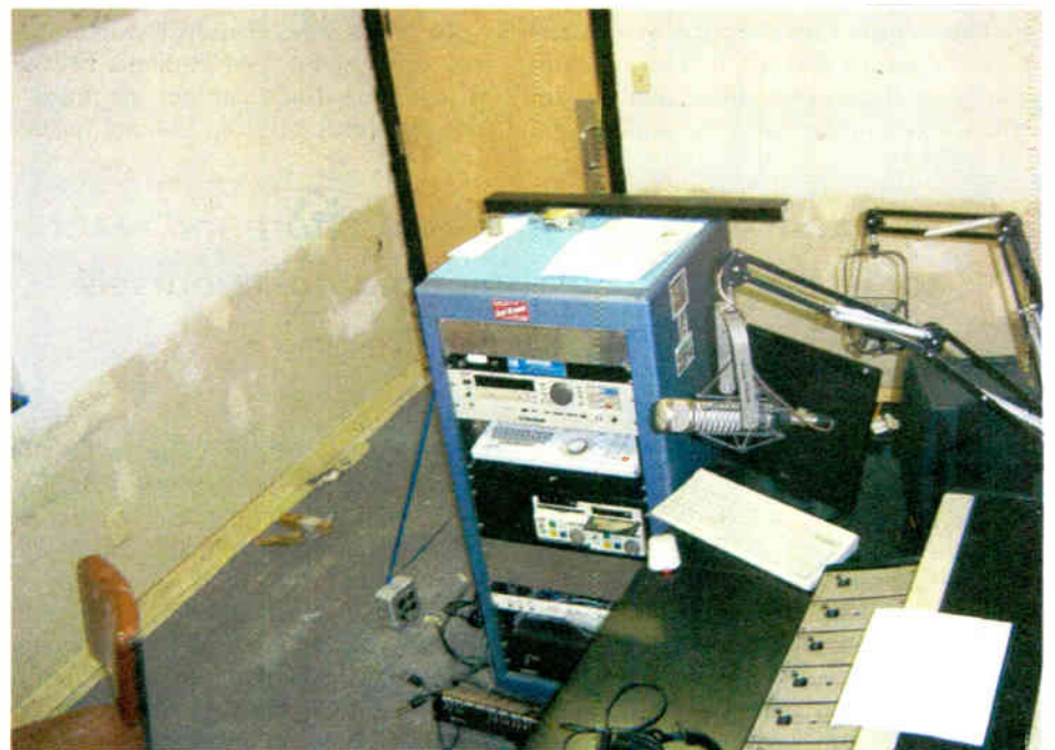
Because on-air audio still went through the room under construction, it was mandatory that certain equipment remain. There was a continuous two-foot stack of gear and wiring in the center of the construction,' said Slentz.
