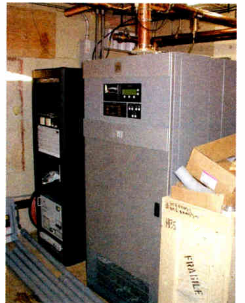
The Nautel V10 during installation at KJNP(FM). The site is on Ester Dome west of Fairbanks, Alaska.
