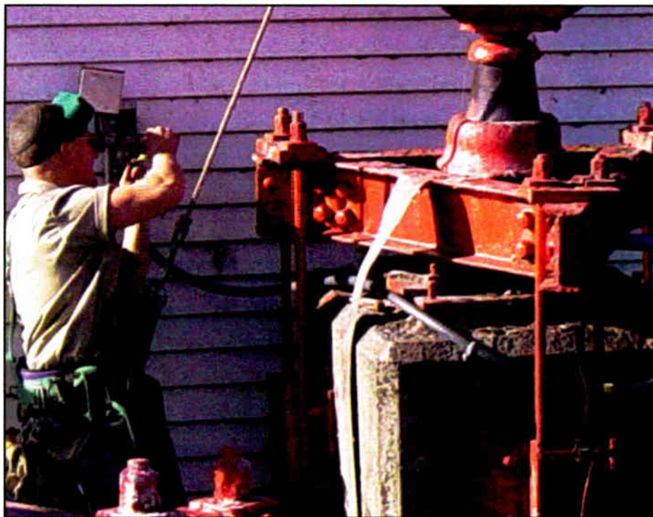
Nick Berg is shown in 2003 working on a lighting circuit at the base of the tower for WMCA(AM), New York. He was replacing a conduit to the tower in the Meadowlands in New Jersey.
