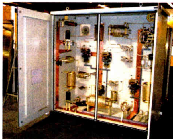
DIRECTIONAL ARRAY ANTENNA TUNING UNIT GAITHERSBURG, MD
