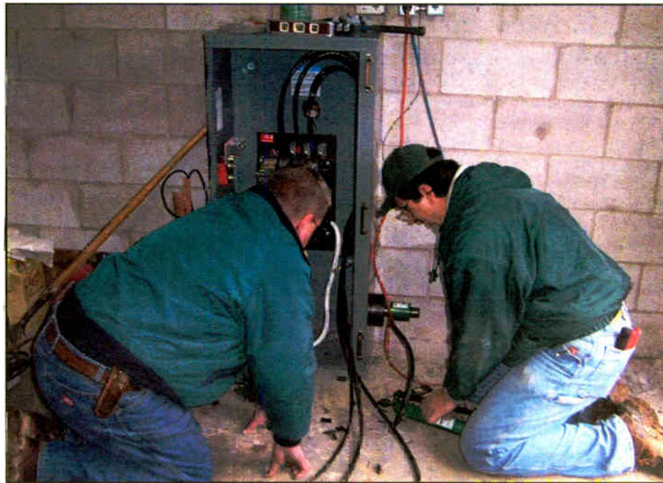
Preliminary installation work is done inside the WXPR transmitter building on the automatic transfer switch.
