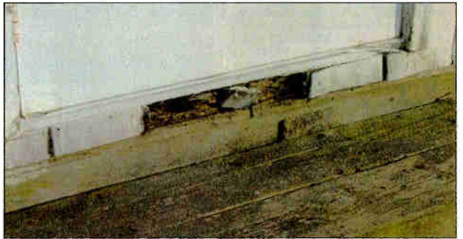
Fig. 2: Don't let severe weather of the past winter lead to major site problems. Do a thorough inspection.
