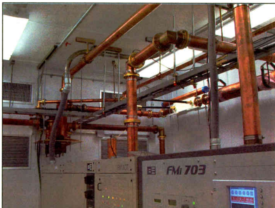
The RF Plumbing With the HD Radio Injector
