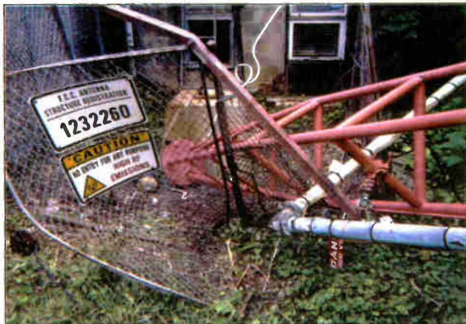
The WHAT tower collapsed in two sections. It broke about halfway up; then the insulator broke and the base gave way.
