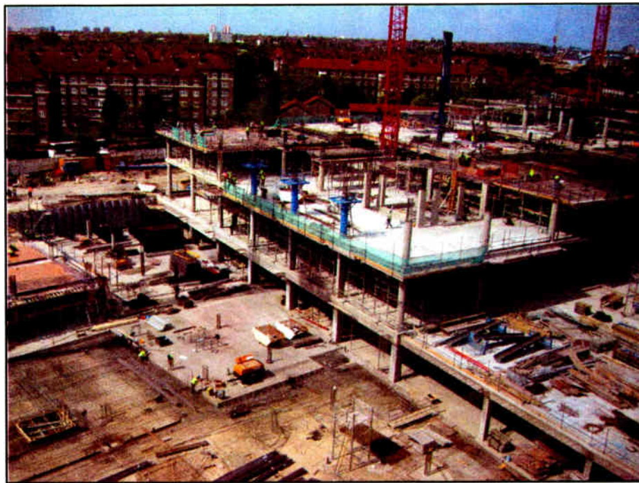
The concrete frame is cast at the BBC's new Broadcasting Centre in West London.
