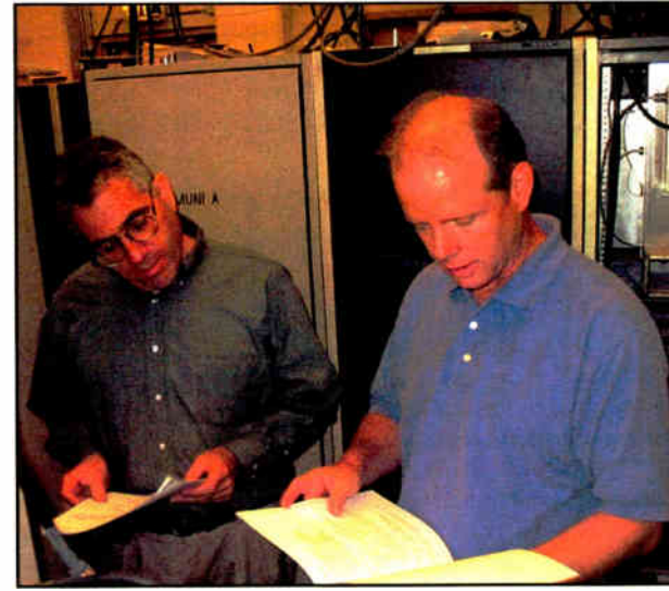
Phil Hartman of KALW(FM) and Dave Agnew of Harris Corp. pause in the transmitter room.
