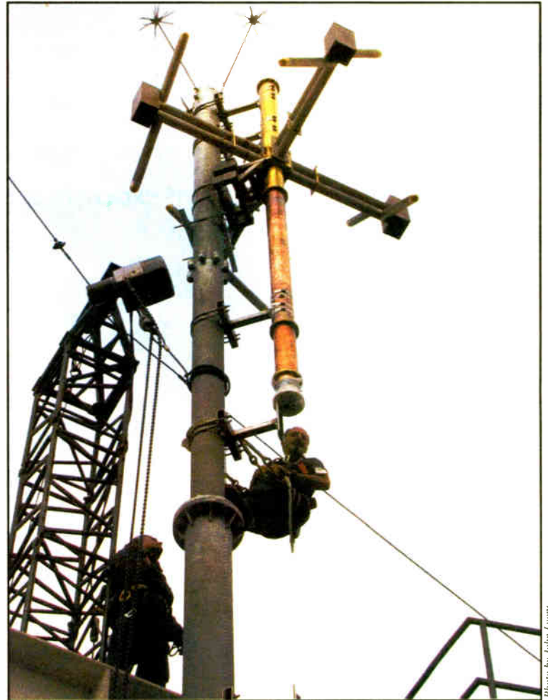
Two employees of Hatzel & Buehler electrical contractors work on the transmission line of the temporary FM master antenna atop 4 Times Square.
