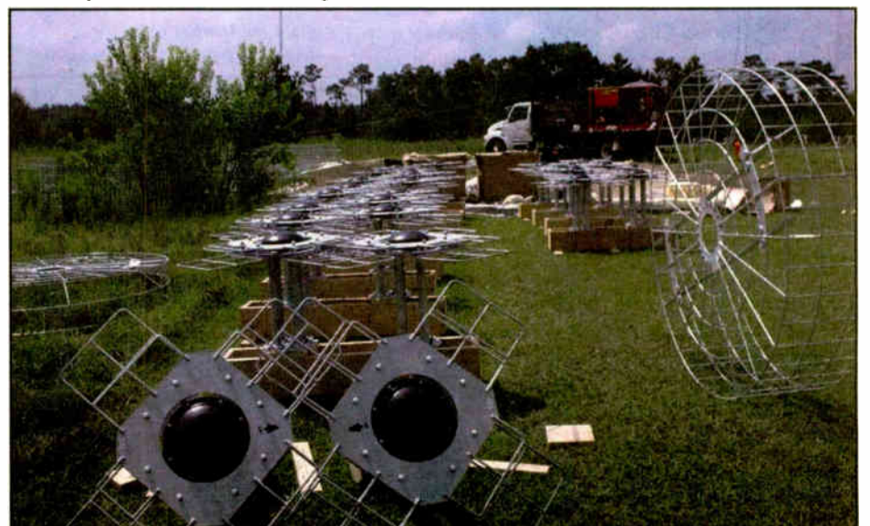
Bays await assembly and installation at the Wilcox Road site in Alabama.
