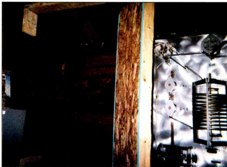
Fig. 2: This wooden barrier protects workers from accidental contact with the RF network on the right.
