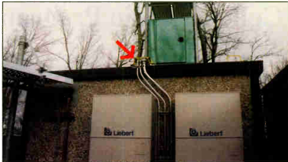
Fig. 3: Also shielded from ice is the cabling conduit (arrow). Dual air conditioners are visible on the wall.
