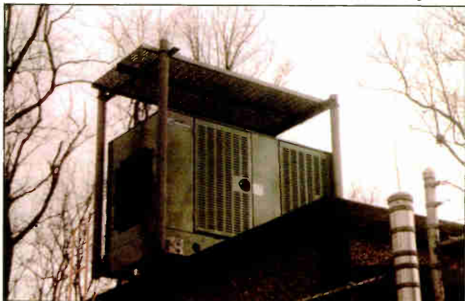
Fig. 2: The generator is on the roof, protected by an ice shield.
