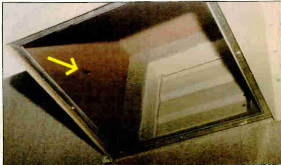
Fig. 2: The arrow shows a wasp trying to enter a transmitter building.
