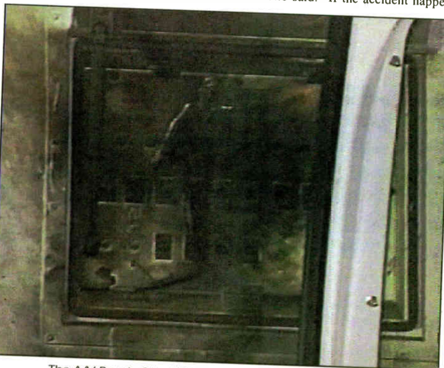
The AV Panel of the WTTG Van After Power Line Contact
