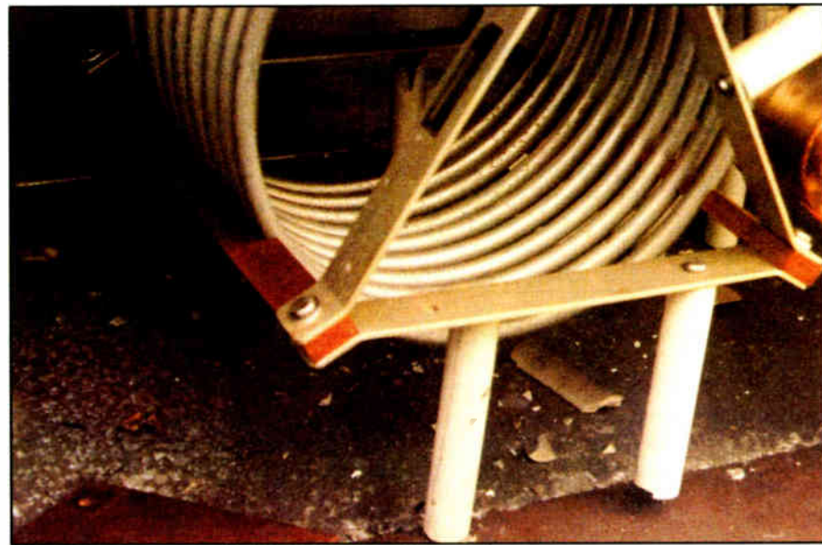
Fig. 3: Check for cracked or broken insulators supporting coils and other components in an ATU.
