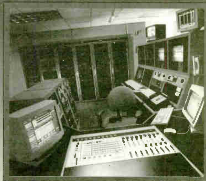
The Master Control Studio, shown right, is one of seven Arrakis studios in Sony's Manhattan network origination center for SW Networks.
