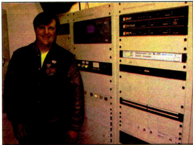
Mike Kernen in the Equipment Room
