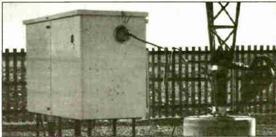
A Properly Installed and Grounded ATU and Tower
