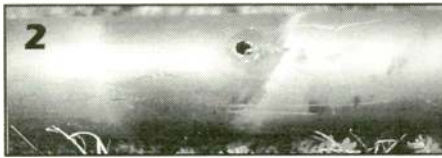
Lightning Damage to Rigid Line Section Causing an Internal Arc
