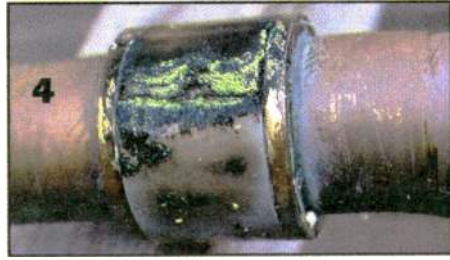
Lightning Damage to Antenna Insulator
