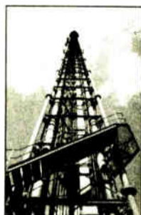
Coaxial Transmission Line
