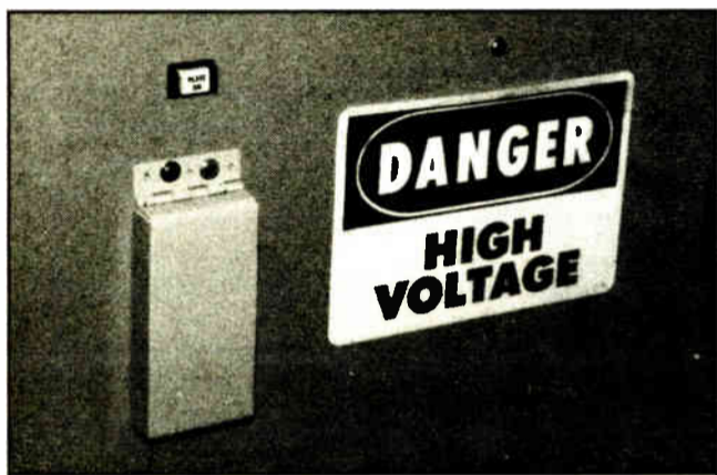
An inexpensive metal cover affixed to the front of this transmitter power supply prevents accidental tripping of the breaker by bumping into it.
