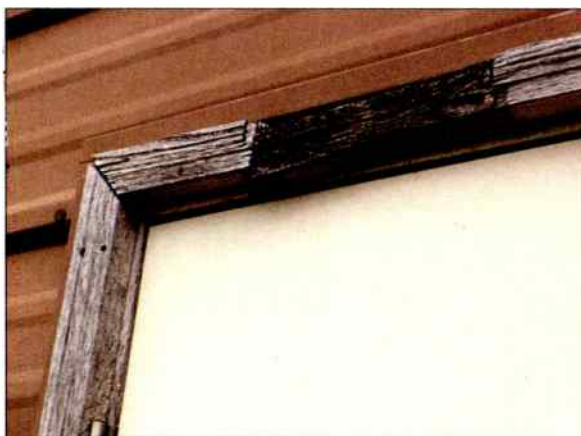
Poor maintenance by the previous owner. A door frame being destroyed due to neglect.
