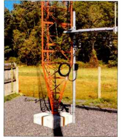
LPU at Tower Base
