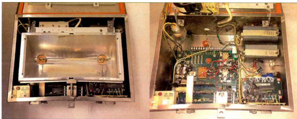
Figure 1 – The old Hughey and Philips SS125 strobe high intensity tower light installed in 1998. There are nine of these boxes on the tower and each box weighs about 70 lbs. On the left side is the flashtube and underneath (right side) are the circuit boards, capacitors, power transformer, etc.
