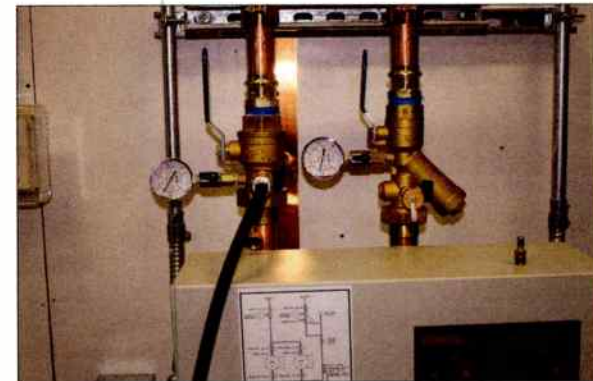
Pump station, showing suction and discharge lines.
