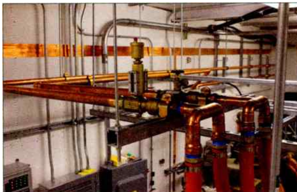
System high point with air purge valve and sight glass.
