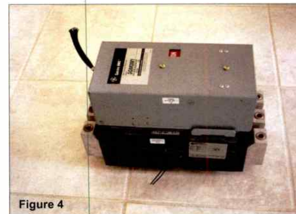
Figure 4 The GE SGMOM1 Motor Driven Device Mounted on the Circuit Breaker
