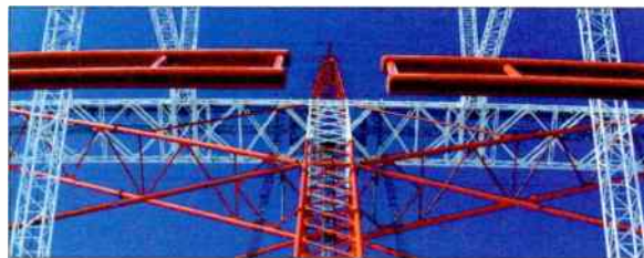
Ampegon Antenna Support Detail
