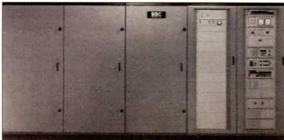
Brown Boveri SK 55, 500 kW Short-Wave Transmitter
