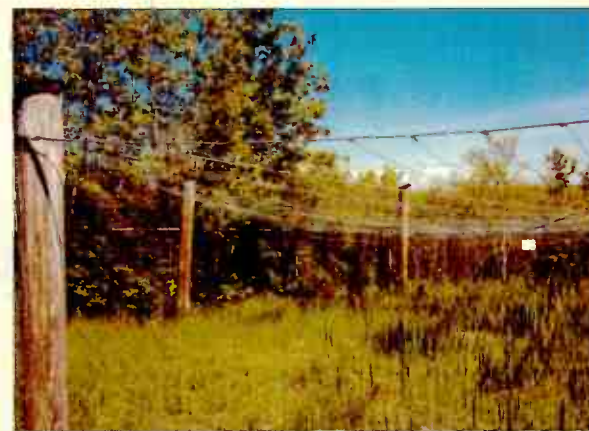
Suspended ground system as it should be.
