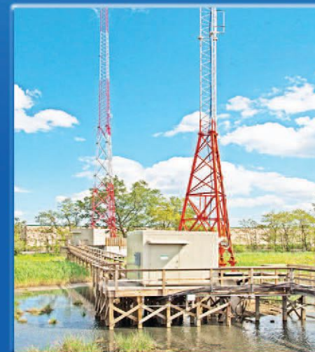
Kintronic supplied pre-fab tuning houses 1380 kHz WKDM - 1660 kHz WWRU Jersey City, NJ
