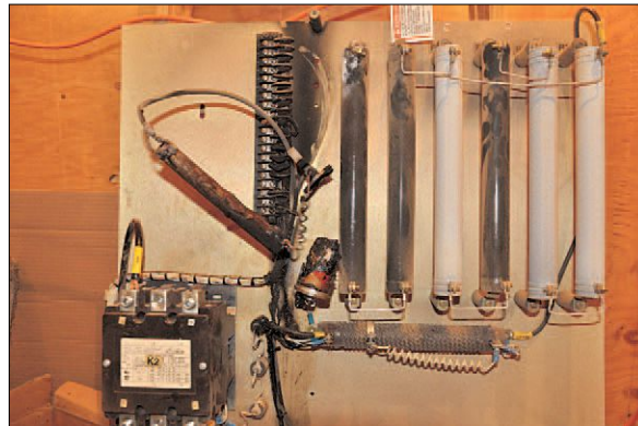
A Badly Burned Panel
