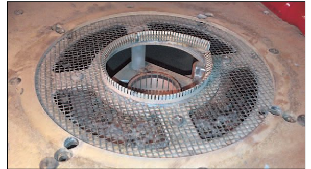
Tube Air Flow Reduced by Debris
