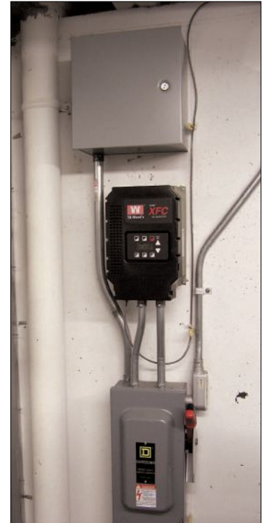
Phase protection on Top, Frequency Drive unit in the middle, and power disconnect on the bottom.
