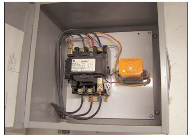
The contactor and Phase Loss module mount inside a 12x12x6 Hoffman enclosure.
