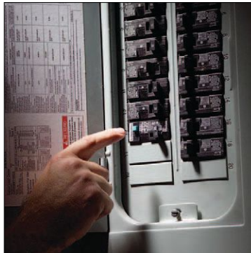
Always check the breakers!
