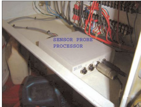
The temperature probes are connected to the Burk processor, installed in Louver control box.
