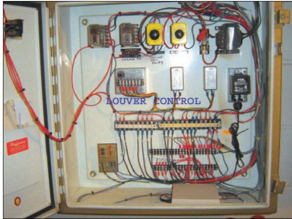
The louver control box with the temperature sensors attached to the box at the bottom.
