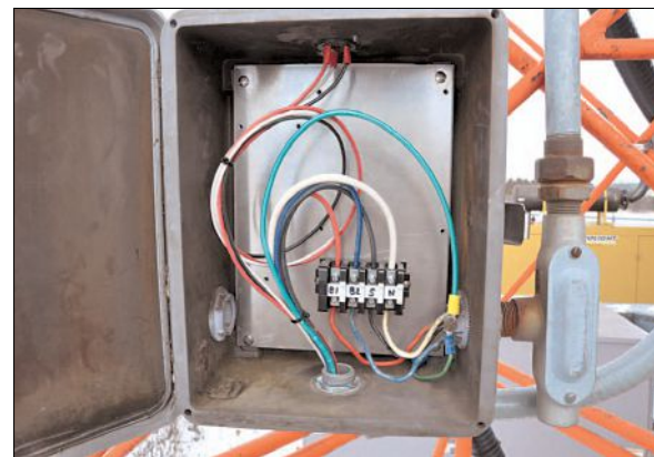
Wiring Junction Box
