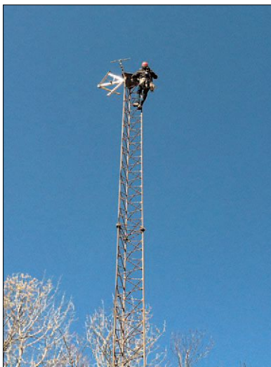
Previous WSUB-LP location on a two-way radio tower.
