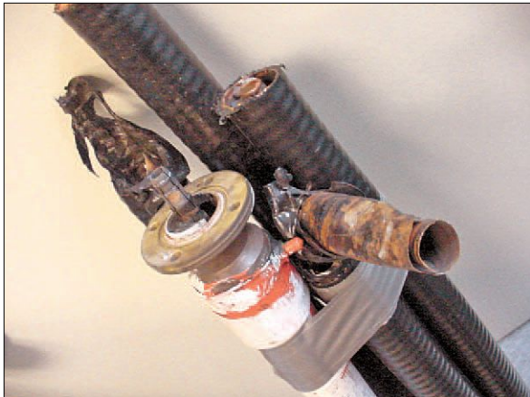
Burned transmission line – a real emergency.
