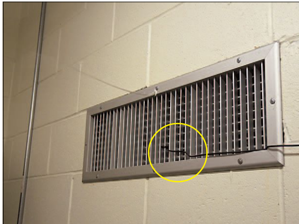
Temperature Probe Installed
