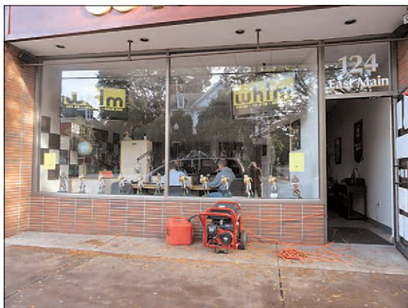
The WHLM studios powered by the Fire Department's emergency generator, per the station's disaster plan.
