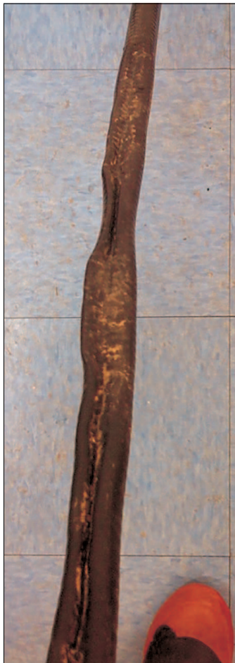
Ice flattened coax. For perspective, note the author's boot tip at the bottom of the picture.
